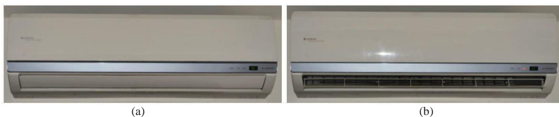
Fig. 13. (Color online) Turning on the air conditioning equipment. (a) Before amd (b) after startup.
